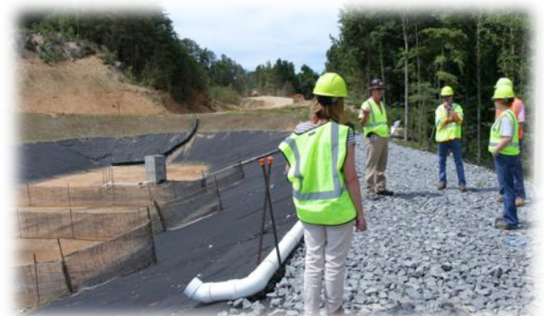
ALDOT shows results of their leadership for stormwater improvements at June 2014 tour of Northern Beltline construction site.
