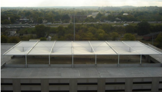
SSA rain collection system over parking. Site plan shows green roof and courtyard that will reduce storm water runoff and save energy
